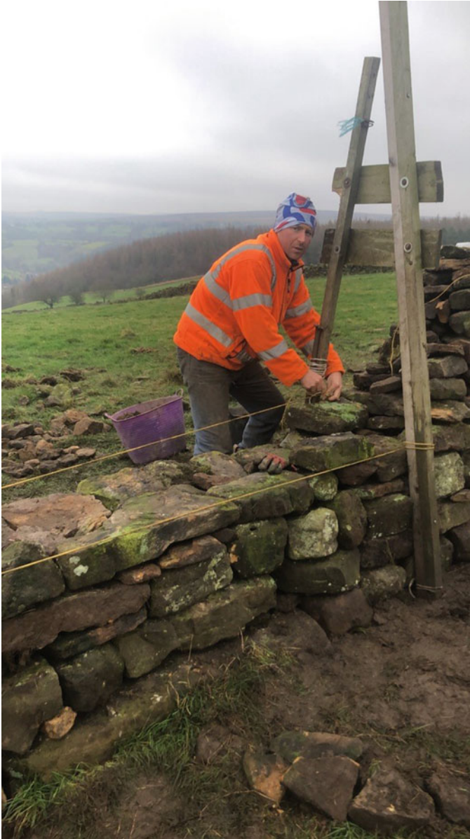
Fig. 5 Calum tying a batter board to set the level of the wall (Source: The author)
