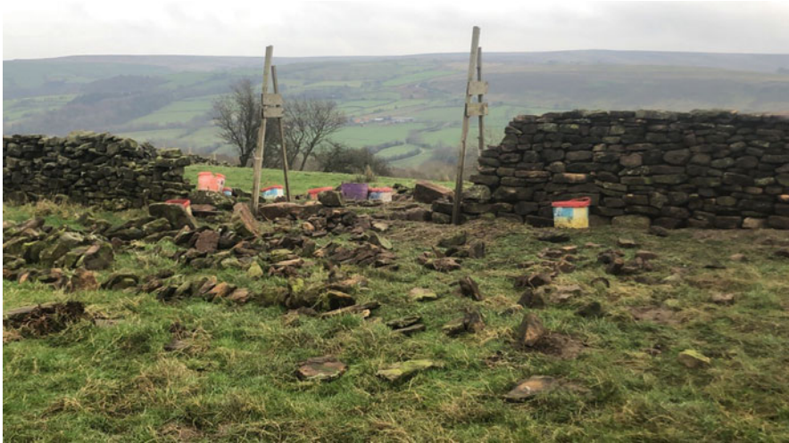
Fig. 3 Batter boards in place on a section of wall in Goathland, North Yorkshire (Source: The author)
