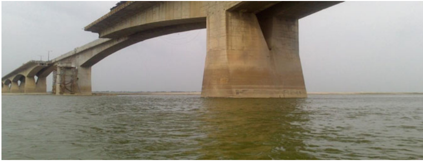
Fig. 13.2 Gandhi Setu with damaged span on River Ganga at Gaye Ghat, Patna
