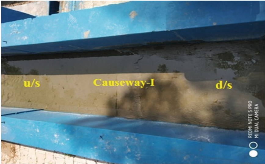
Fig. 32.5 Photogrammetric view of scour around causeway-I
