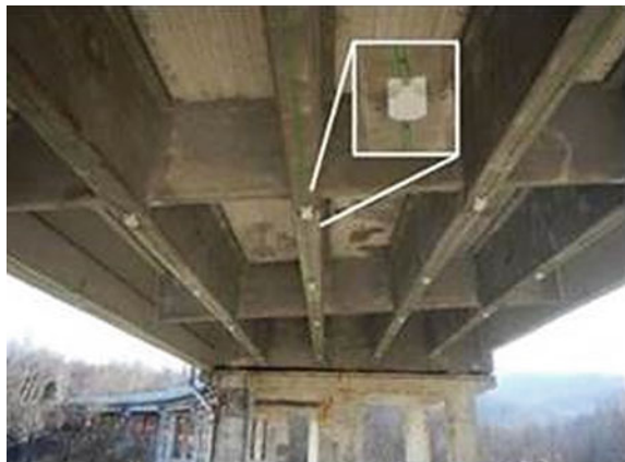
Fig. 5 Cabled network installed on a bridge: a CAN bus connects the sensor nodes
