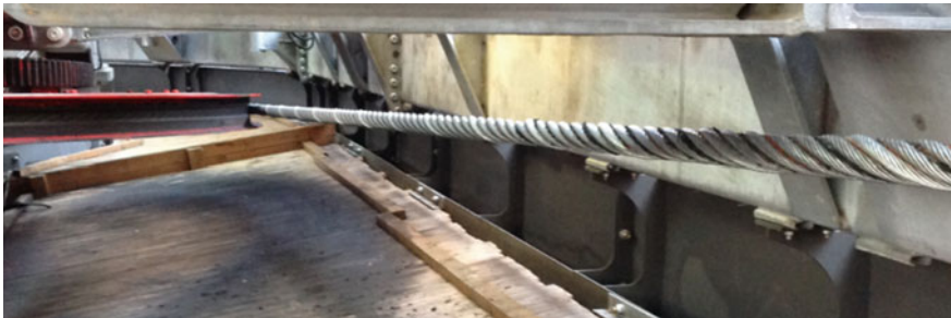
Fig. 6. Photo of a defective section of a rope with a diameter of 48 mm, construction 6 \times 26 (1 + 5 + 5/5 + 10) WS-SPC 1600 B zZ with visual twisting around its axis.
