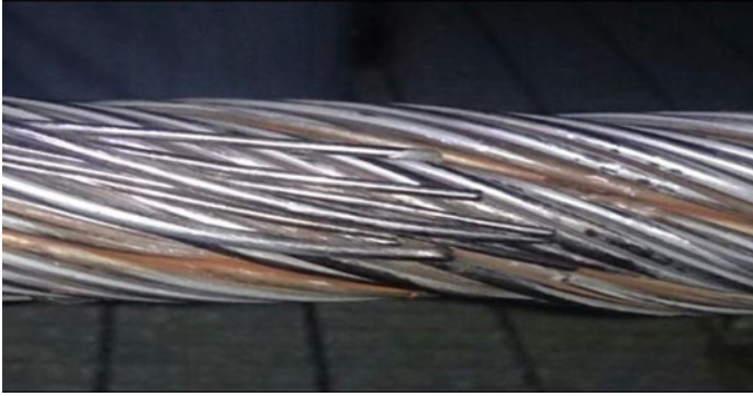
Fig. 8. Photo of a defective splicing section of a steel rope with a diameter of 48 mm, construction 6 \times 26 (1 + 5 + 5/5 + 10) WS-SPC 1600 B zZ with the presence of corrosion of damaged wires of one of the strands.
