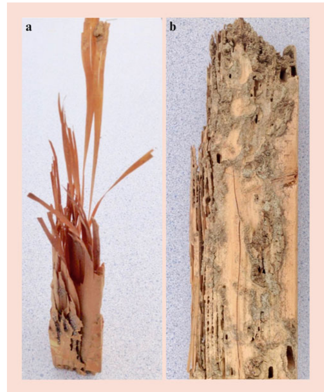
Fig. 4.13 (a) Subterranean termite damage to a “2x4” structural wood member. Note the characteristic “muddy” appearance of the gallery which resembles dried oatmeal and results from termites packing fecal material and soil particles into galleries. Subterranean termites feed with the grain of wood – removing earlywood xylem tissue, leaving behind denser latewood. (b) Subterranean termite damage. (Note the laminated appearance of the wood resulting from consumption of softer earlywood, leaving the denser latewood untouched)
