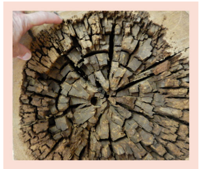
Fig. 4.3 Brown rotted wood decay from the collection of Holzforschung München, Technical University of Munich, shown with the first author's hand for scale. The interior wood is in an advanced stage of brown rot degradation. In advanced stages of decay, the wood is brown in color and often has a cross-hatched or cubical appearance
