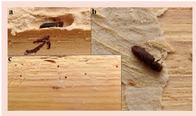
Fig. 4.15 Powderpost beetle damage by the genus Lyctidae: (a) A lyctid beetle resting in an exposed pupal chamber, after maturation from the larvae into an adult, and just prior to what would have been the emergence flight. (b) A dead adult lyctid beetle on the surface of wood debris. (c) The appearance of infested wood after powderpost (lyctid) beetle larvae has bored through the wood and the adults have emerged through the flight hole. The upper half of the panel has been surfaced with a razor to reveal the galleries of the larvae below the surface of the wood. Comminuted wood powder produced by the larvae within those galleries is also present on the surface of the wood
