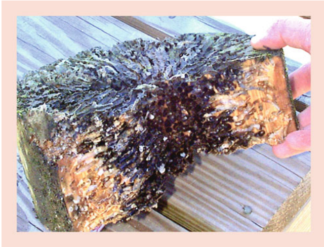
Fig. 4.21 Tightly packed galleries of shipworms in oak wood piling. This piling in the cold coastal waters of Maine USA was attacked and completely riddled by shipworms over a one-year period until failure occurred. Typically, after entering the wood wherever access is permitted, shipworms will re-orient their galleries to align with the wood grain. In this case, however, the number of animals boring into the wood did not permit gallery realignment, and the shipworms burrowed directly to the center of the piling until the piling was weakened enough to fail
