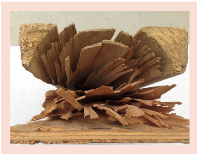
Fig. 4.16 Carpenter ant damage to a “2x6” support and plywood sheathing (cross-sectional view). The “2x6” pressure treated member was poorly treated with preservative in the interior heartwood and extensive carpenter ant damage occurred in this relatively untreated heartwood. The attack occurs in a lamellar manner, with the denser latewood remaining as the lower density early is removed. (Note removal of wood with the “sand-paper smooth” appearance of galleries and also the lack of fecal material and soil particles (mud). The sapwood of the “2x6” member at the top left and right is penetrated better than the heartwood by the pressure treatment, and hence the sapwood has not been attacked)
