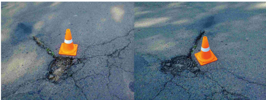
Fig. 3 Stereo-pair of two photographs of a traffic cone against the background of damage to the road surface
