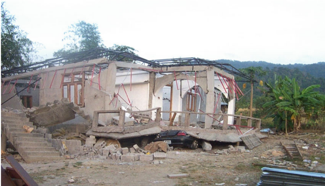
Fig. 1.12 Earthquake at Kalyanpuram, South Andaman, India. This Sumatra-Andaman earthquake—the Great Tsunami—of December 26, 2004, was of magnitude 9.1 causing Grade 5 damage to a newly constructed RCC framed structure (photograph taken on January 09, 2005). The earthquake rendered total collapse of the ground floor
