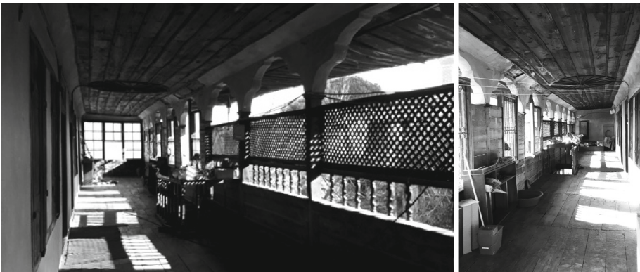
Fig. 5. The open gallery of the first floor from outside and inside. Photos: Alicja Maciejko, Interiors (2020) [2].
