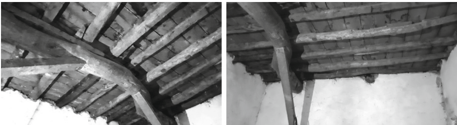
Fig. 11. Structural beams and floor decking, ceiling, underside view. Interiors (2019). Photos: Alicja Maciejko [2]
