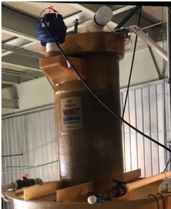
Fig. 5 The gas-stripping tower is mounted on the top of the moving bed bioreactor
