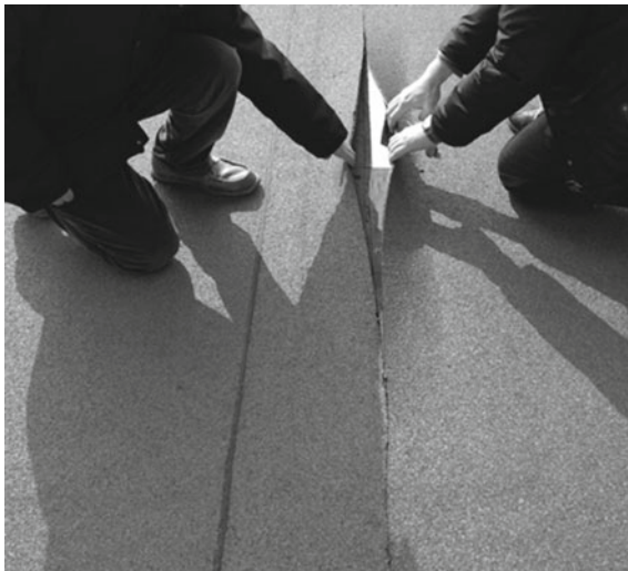
Fig. 4 Cracking due to thermal contraction before precompression destabilization phase. Cracking is favored by reinforcements anisotropy and the continuous joint between panels oriented in the longitudinal direction of the sheet
