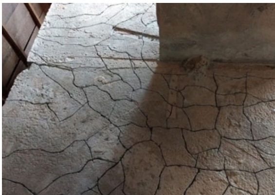
Fig. 4 Map cracking on the surface of the pile cap block
