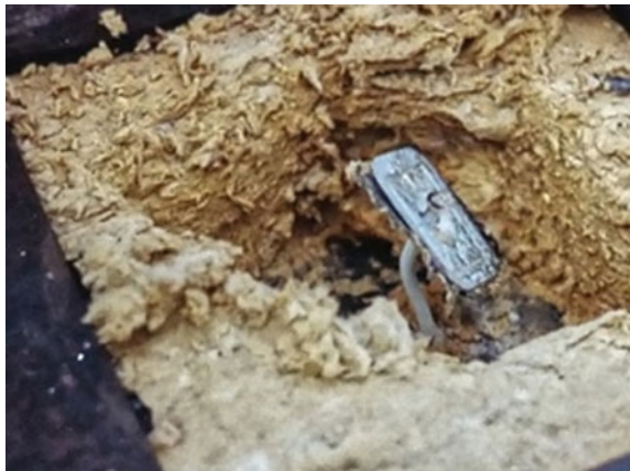
Fig. 10 Deformation of the mechanical fixing shaft due to direct load
