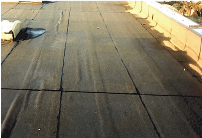
Fig. 3 Corrugations due to gap presence between insulation panels
