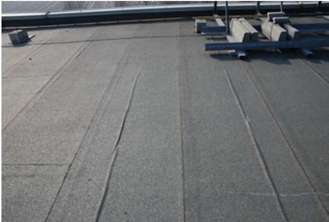
Fig. 6 Longitudinal corrugation due to relaxation of the membrane. Reinforcement was polyester, reinforced with longitudinal fiber glass, therefore anisotropic
