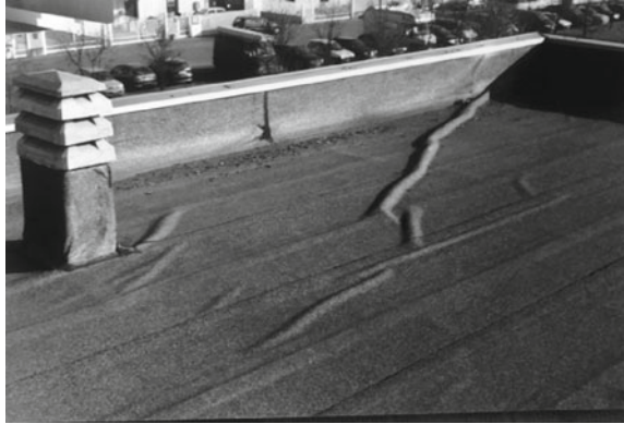
Fig. 7 Corner corrugation, horizontal and vertical
