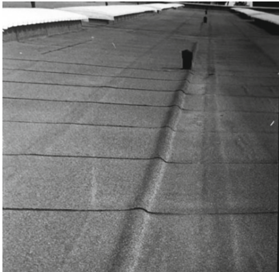
Fig. 5 Transversal wrinkling due to detachment from orthogonal edges to the direction of sheet installation
