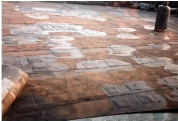
Fig. 9 Refurbishments in correspondence of mechanical fixing shafts, due to insufficient compressive resistance of the insulation panels
