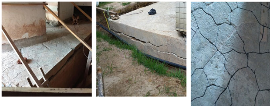
Fig. 1 Cracking process found in pile caps investigated
