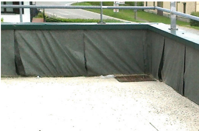
Fig. 8 Corrugations due to floor contact with the waterproof cuff. Wrinkles have diagonal shape, pointing down. Overlaps are detached
