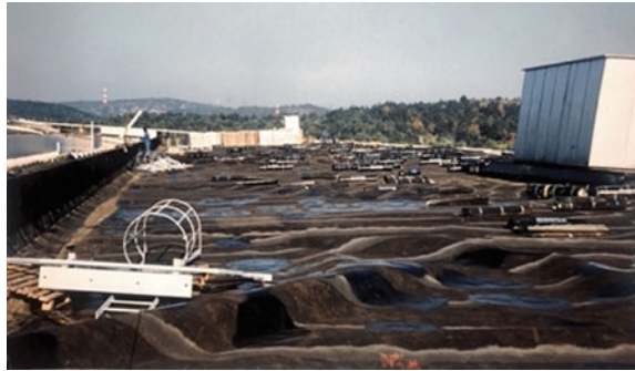
Fig. 12 Urgency ballasting of a membrane detached by the wind
