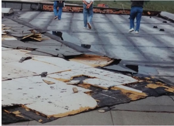
Fig. 13 Dislocation due to wind for insufficient adherence of the membrane to the support
