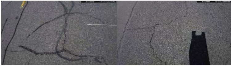
a) Cluster 0 (multi-directional cracks)
