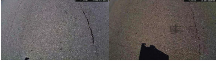
b) Cluster 1 (longitudinal cracks)
