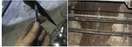
Fig. 1. Engineering problems of subway tunnel in weathered argillaceous siltstone
