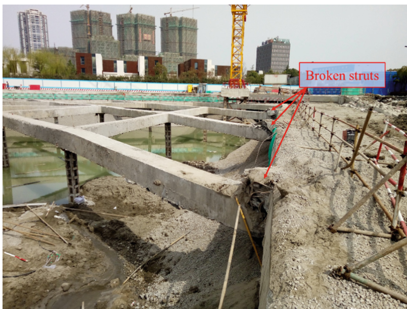
Fig. 3. Picture of the failed deep excavation
