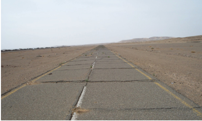
Fig. 1. Tayma-Tabuk abandoned road (Saudi Arabia); severe distress.
