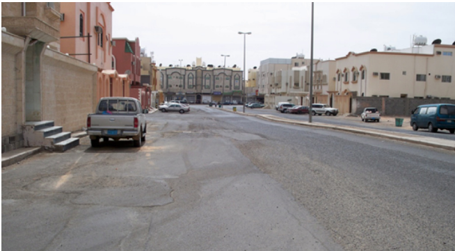
Fig. 3. A road under frequent maintenance due to expansive soil, Al-Rowda district, Tabuk, Saudi Arabia
