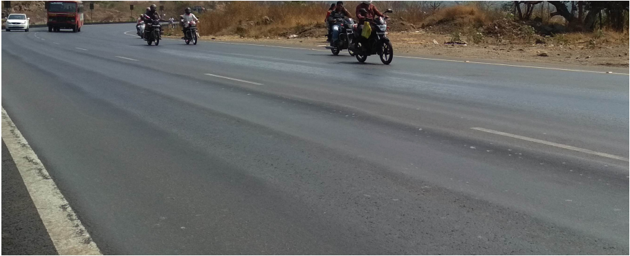
Fig. 2. Rutting failure on NH-4 Near Satara
