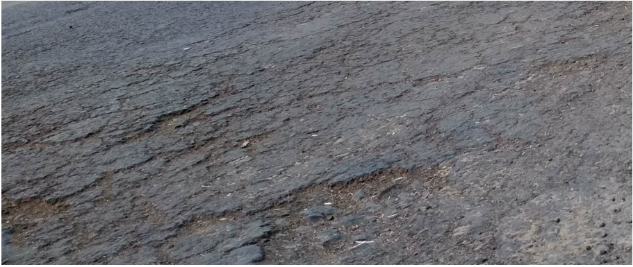
Fig. 3. Fatigue failure on NH-4 Near Satara
