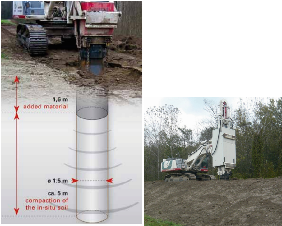
Fig. 22. Impulse Compaction embankment improvements for a high water protection dam in Austria
