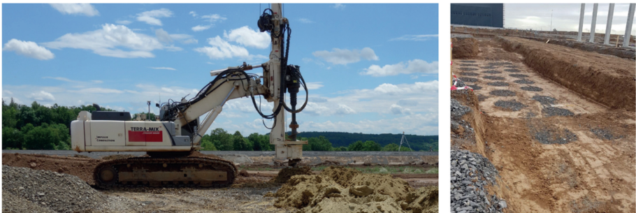
Fig. 16. Impulse compactor with drilling attachment in Sachsenheim (left), and resulting gravel columns (right).
