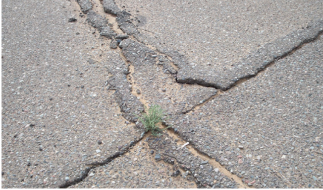
Fig. 2. Close-up view of localized distress (Tayma-Tabuk Road, Saudi Arabia)
