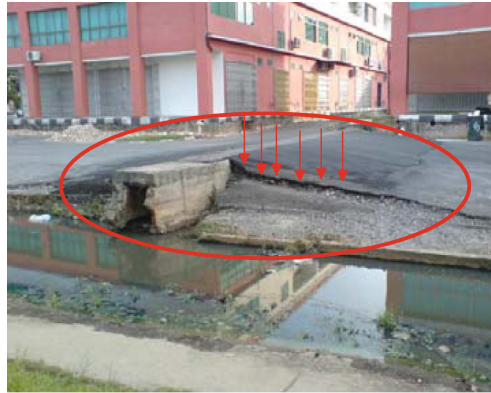
Fig. 1. Hazardous settlement of approach road with peat ground subsidence in Sibul, Sarawak, Malaysia (Kolay et al. 2011)
