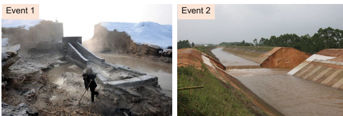
Fig. 1. Failures of soil embankments from the field observation (a) Event 1 occurred in Xinjiang, China, February 2013 (Chen 2013) and (b) Event 2 occurred in Guangdong, China, May 2014 (Yu 2014).
