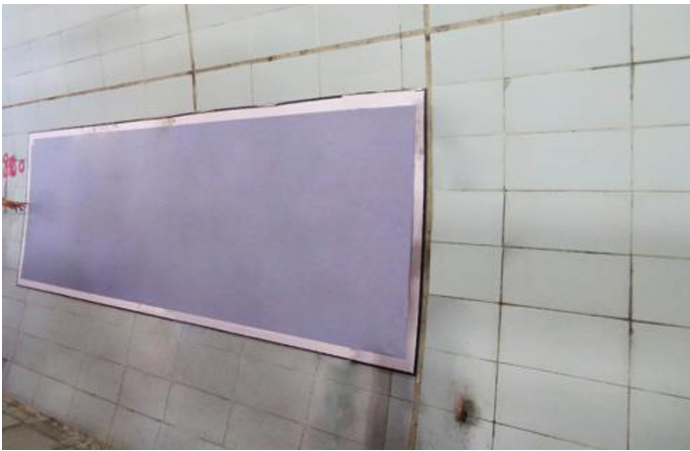
Fig. 14. installation position of crack plate on side wall of three lane tunnel.
