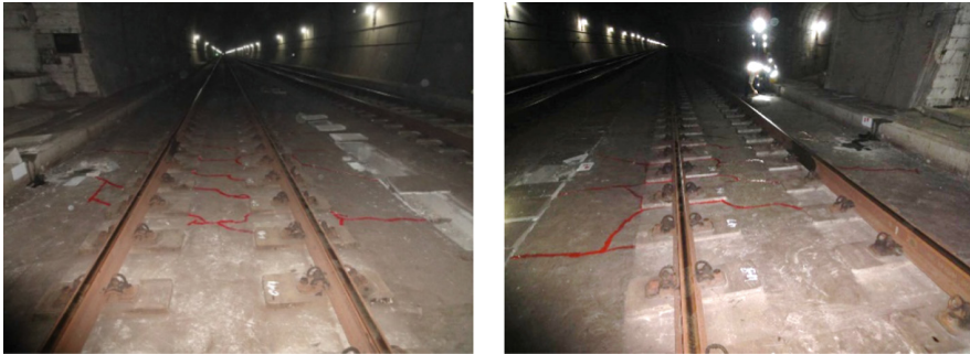
Fig. 2. Cracking of invert filling and track slab.
