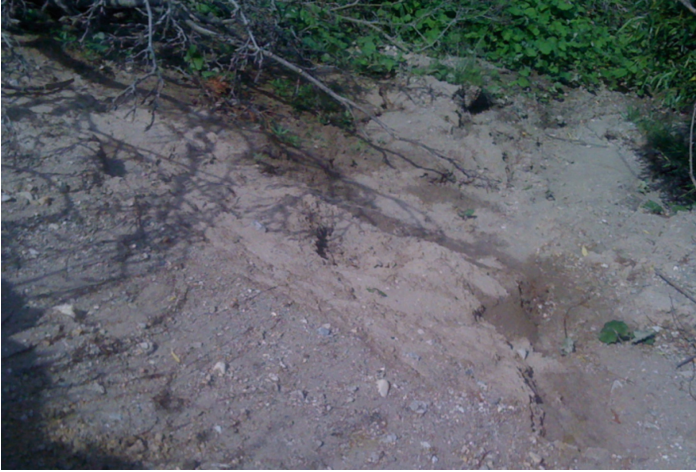
Fig. 7. Piping and mudflow was observed on bank-slope surface of Thames River at the study site (picture taken by Ron Xia on June 11, 2015).
