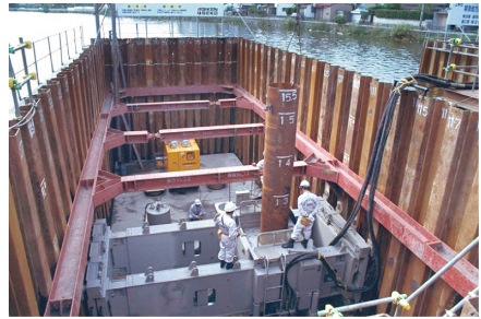
b) System that a piling machine stretches its arm to sheet piles to obtain reaction force (OS1-3)
