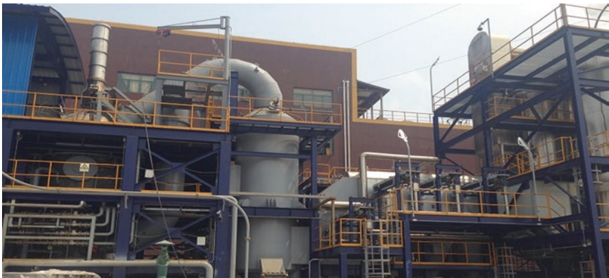
Fig. 39.5 A typical incinerator
