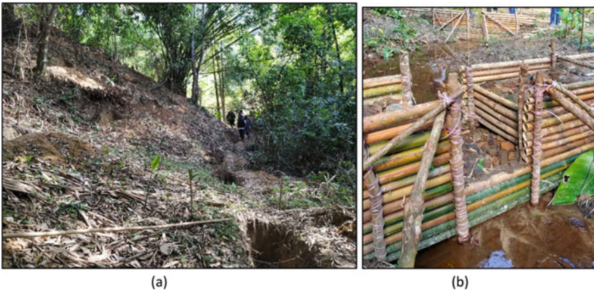
Fig. 9.4 a Trenches excavated at hill slope, and b Bamboo check dam constructed in stream
