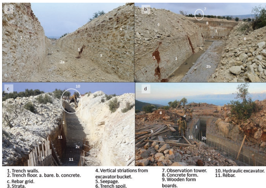
Fig. 17.5 (a) Syrian Kurdish trench excavated in horizontally bedded limestone with marls using a machine. (Modified from Vatan 2018). (b) Syrian Kurdish trench in chalky limestone with marls dug using a mechanical excavator prior to a concrete floor being poured. The white oval shows an OT. (Modified from Yeni Safak 2018b). (c) The white oval shows a tracked excavator digging a Syrian Kurdish trench with a small 305-mm bucket. (Modified from Takvim 2018). (d) Concrete-lined Syrian Kurdish defensive trench in limestone on Mount Bursaya. (Modified from Southfront.org 2018)
