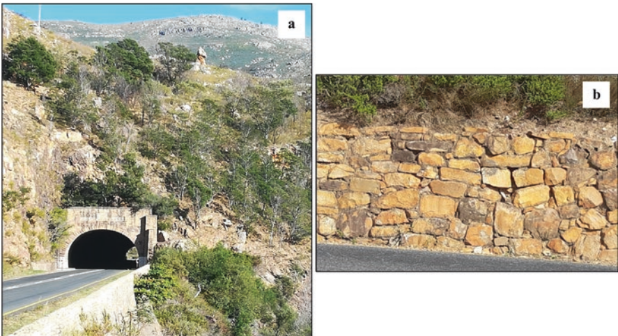
Fig. 10.7 (a) Tunnel and (b) retaining wall built by Italian POWs in Du Toitskloof Pass, South Africa. Note the difficult terrain in (a) through which the road was built
