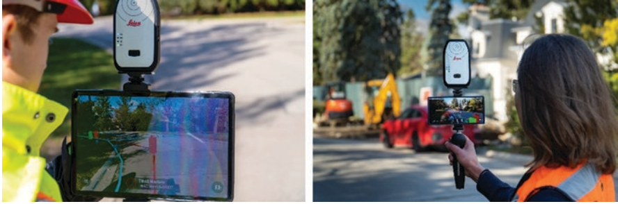
Fig. 9.8 Using smart devices with a location sensor to visualize underground infrastructure such as buried pipes and cables for construction: (a) with a tablet and (b) with a smart phone. (© vGIS Inc. All rights reserved)
