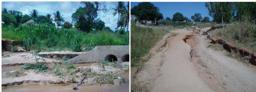
Fig. 1 Access roads destroyed by erosion
