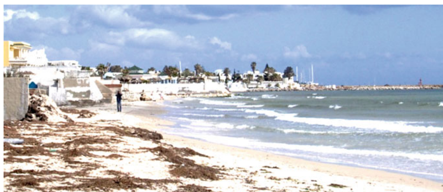
Fig. 15 The decrease in beach surface south of Port El Kantaoui. [1]. As this picture shows, the holiday resort located south of Port El Kantaoui settled directly on the maritime coastal area (DPM), destroying the dune edge and resulting in the reduction of beaches that, in some places, have completely disappeared
