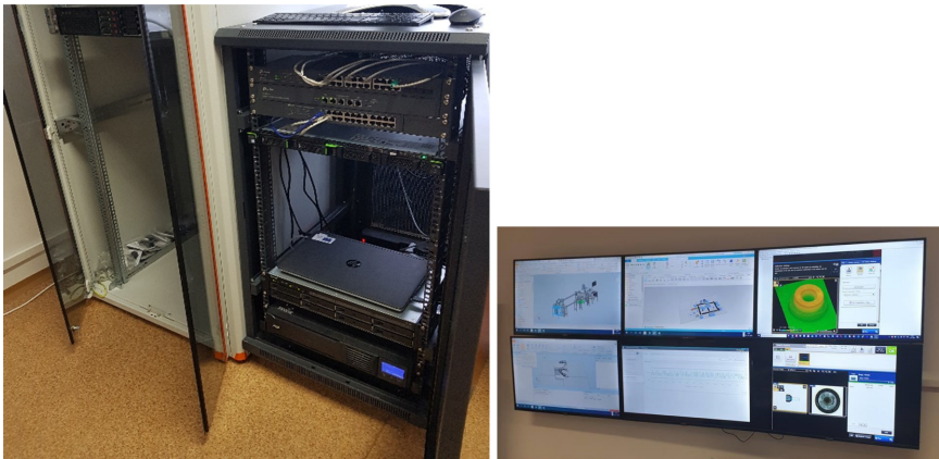
Fig. 11. Rack servers HP Proliant and Fujitsu Primergy (Left), Visualisation of data for monitoring and error localisation (Right).
