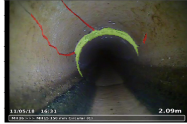
(b) Photo example with annotations: defective transverse joint and axial cracks without discontinuity
