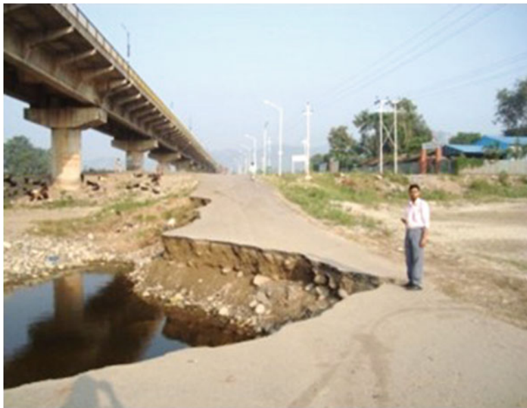
Fig. 8.14 Development of a new avulsion channel, below Chandi bridge during the 2010 flood (field survey, October 2010)
