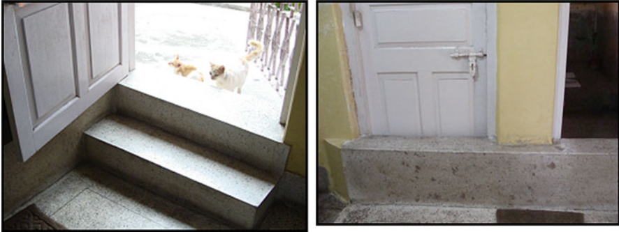
Fig. 25.14 Adjustments for waterlogging: Relative lowering of the adjoining plots causing surface runoff inflow into the ground floor of the houses, Ward no. 123. (Source: Photographs taken by the authors 2017)
