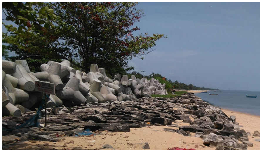
Fig. 7.9 Maintaining the coastal stability ; tetra-pods are deployed to protect the coast after eroding the previous gabions – view from Koyilandi . (Photograph taken by author/s)
