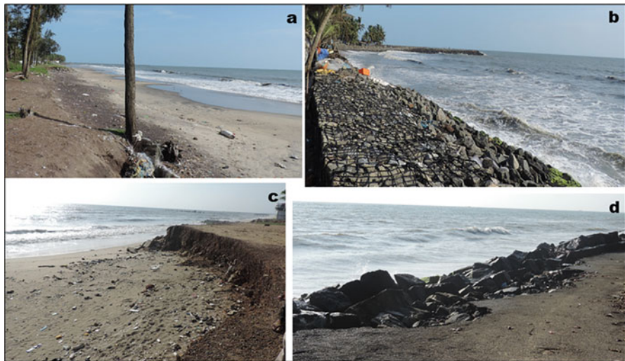
Fig. 7.8 Coastal protection measures and associated coastal erosions; (a) Gotheeswaram beach, (b) Kothi , (c) Kuttichira beach, and (d) Konad . (Photograph taken by author/s)
