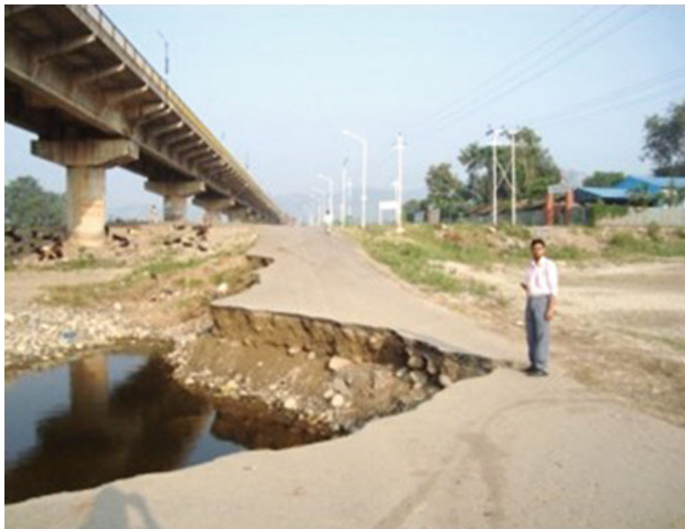
Fig. 8.14 Development of a new avulsion channel, below Chandi bridge during the 2010 flood (field survey, October 2010)
