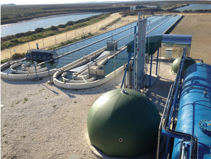
Fig. 4 Raceway ponds of All-Gas project in the El Torno treatment plant in Chiclana, Spain (EU FP7 All-Gas project). Source: AQUALIA
