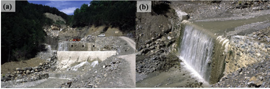
Fig. 7 (a) Construction of new check dams in the lower stretch of the Arás ravine (Upper Gállego basin), following the collapse of most of check dams during the extreme flood of August 1996; (b) New check dam in the lower course of the Arás ravine (Upper Gállego basin). It was constructed after the collapse of most of check dams during the extreme flood of August 1996 (Photos JM. García-Ruiz)
