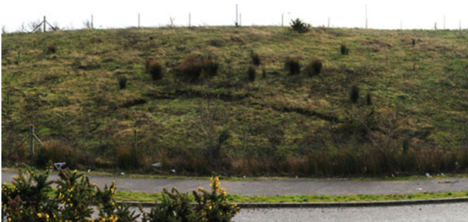
Fig. 6 A27 Polegate/bay tree lane FRS trial; note arcuate back scar indicating slope failure [6]
