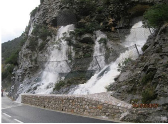
Fig. 17 Situation of PK 158,140 MI produced by heavy rains on rocky slope (upstream) performed the performance
