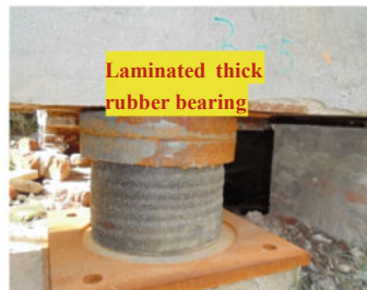
(h) The installed thick rubber isolator.
