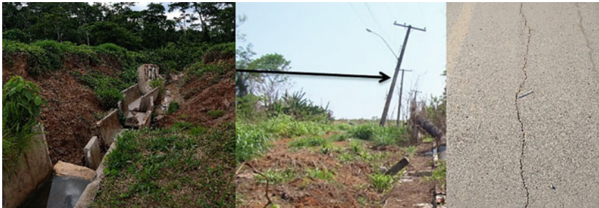
Fig. 1 Damages to infrastructure due to expansive soils in Rio Branco city
