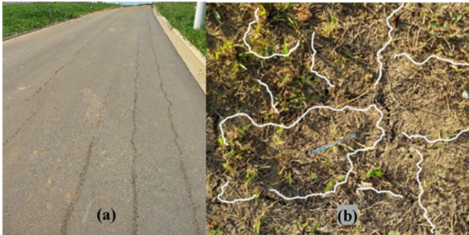
Fig. 5 a Typical longitudinal crack in the site study and b occurrence of cracking in roughly polygonal patterns at the studied site
