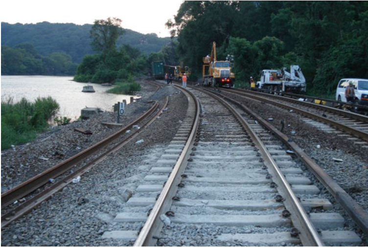
Fig. 2 Track conditions at the point of derailment [8]
