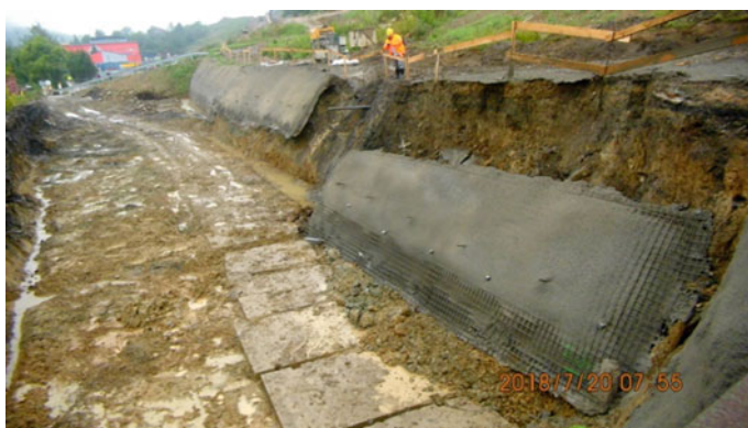
Fig. 13 More than a week open unsecured excavation and one-day rain
