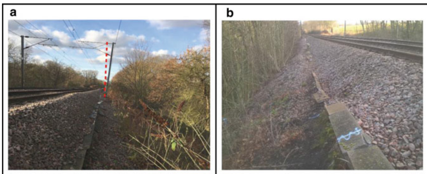
Fig. 5 a—Thick ballast shoulder spilling downslope and leaning OLE mast (looking west). b—Drop in cess level with associated ballast thickening and adjacent track dip (looking east)
