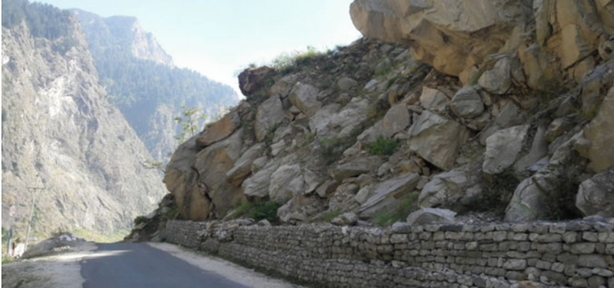
Fig. 7 Stretch with large boulders and open pores. Note the damage to the non-engineered handmade gabion wall
