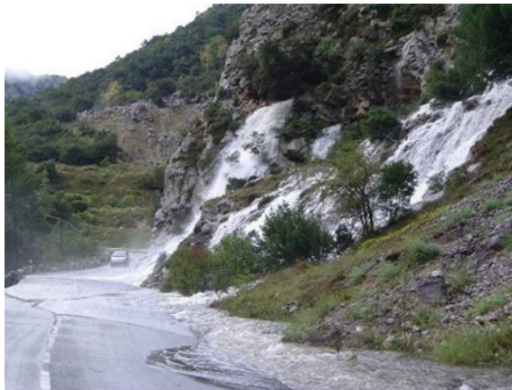
Fig. 1 Situation of PK 158,140 MI produced by heavy rains on rocky slope (upstream) without acting
