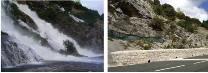
Fig. 9 Situation of PK 158,140 MI produced by heavy rains and situation of PK 158,140 MI with the finished stonework (national roadside)
