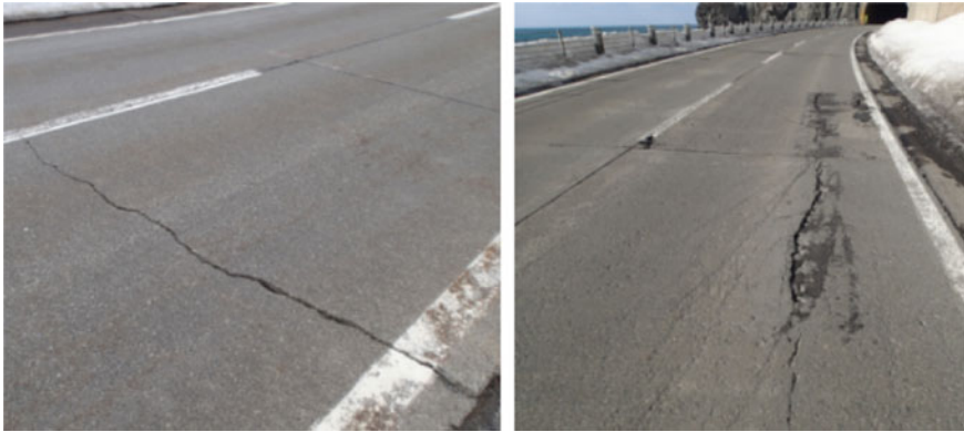
Fig. 3 Structural damage in the Co slab (Left: transverse cracking, Right: longitudinal cracking)
