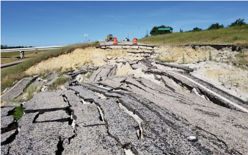
Fig. 1 Condition of slope in June 2019
