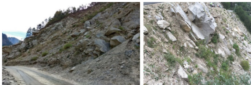
Fig. 3 Slopes adjoining the highway at Govindghat with boulder-soil matrix. The photo on the left shows strata above road level, and the one on the right shows the strata below road level
