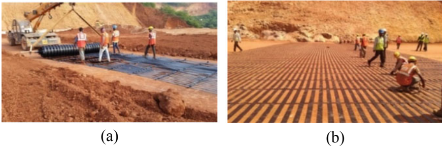
Fig. 11 Geogrid activities: a Unrolling of geogrid; b stretching and fixing of geogrid
