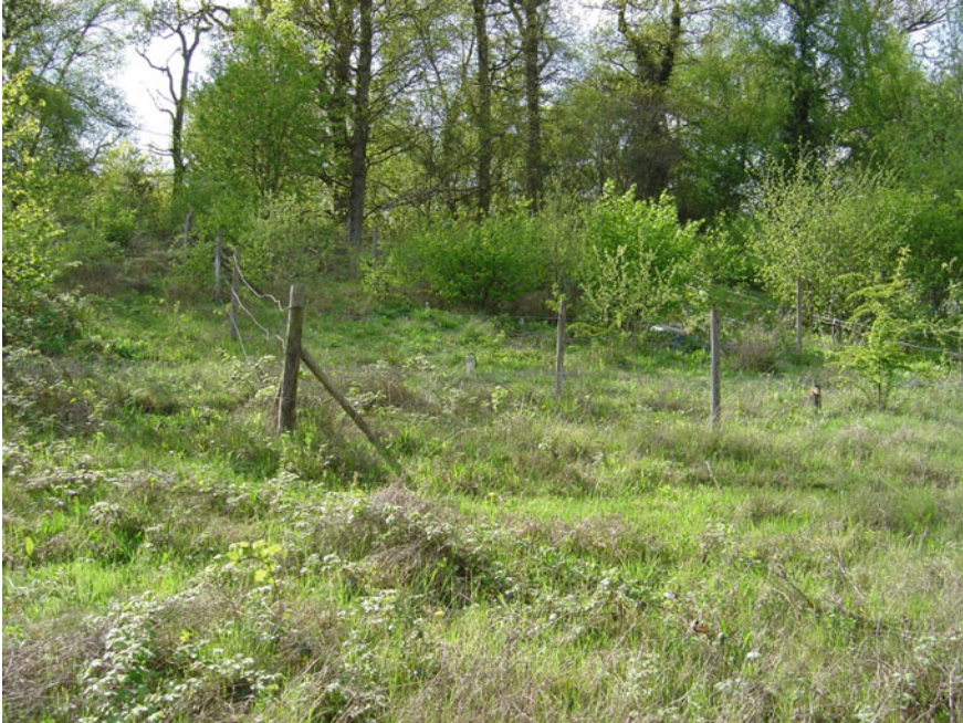
Fig. 2 Instrumented site at Newbury, looking upslope from close to the toe of the cutting. Picture was taken in April 2015. The slope is now more heavily vegetated than shown here
