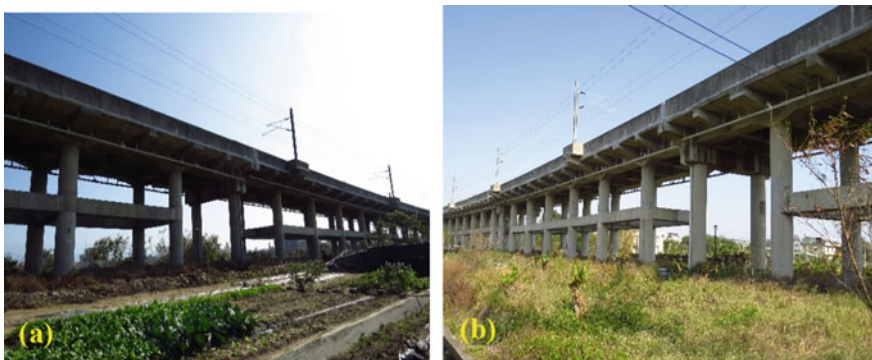
Fig. 4 Rail bridge panorama images: a view from the northwest; b view from the southwest
