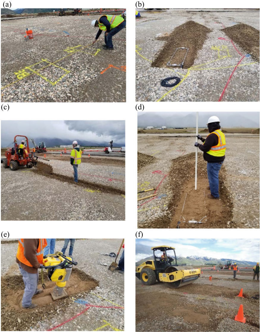
Fig. 5 BE field sensor installation procedure: a marking sensor location; b removing constructed aggregates and placing BE field sensor; c preparing the trench for cables; d measuring the depth of placement of BE field sensor; e preliminary compaction using a plate compactor; and f final compaction after sensor installation using a vibratory roller compactor
