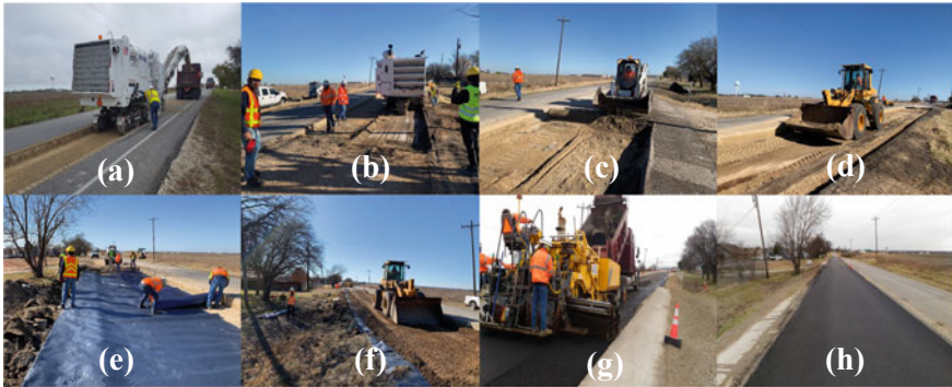
Fig. 2 Construction sequence of flexible pavement using wicking geotextile: a milling, b excavation, c leveling, d compaction, e laying of the wicking geotextile (H 2 Ri), f laying of base course, g asphalt overlay, and h final pavement section
