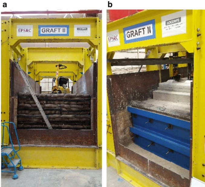
Fig. 3 a Construction of the GRS-RW test specimen and b completed structure prior to cyclic loading for concrete slab track
