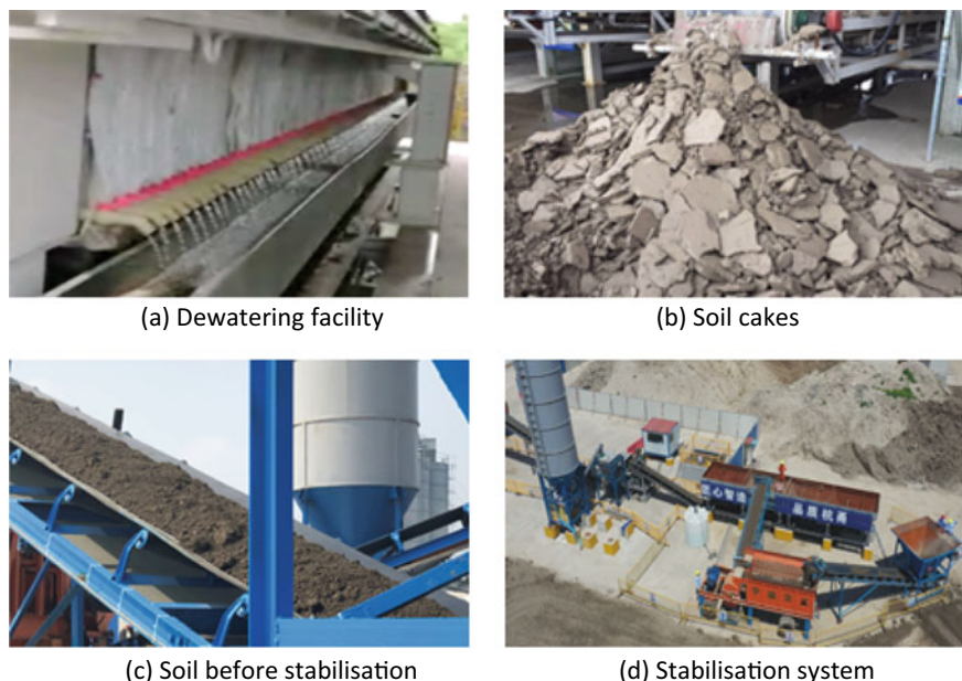
Fig. 9 Slurry treatment plant in Ningbo. a Dewatering facility. b Soil cakes. c Soil before stabilisation. d Stabilisation system
