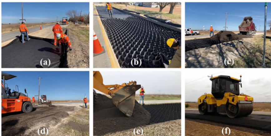
Fig. 2 Construction sequence: a placement of geotextile, b placement of first geocell layer, c placement of RAP, d compaction of GRRB layer, e placement of second geocell layer, and f final surface layer
