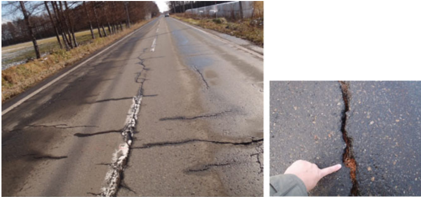
Fig. 1 Deformation due to frost heave of pavement surface
