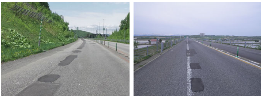
Fig. 1 Damaged porous asphalt (PA)
