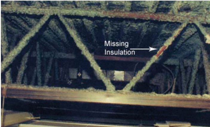
Fig. 5.12 SFRM adhesion failure (localized) [25]
