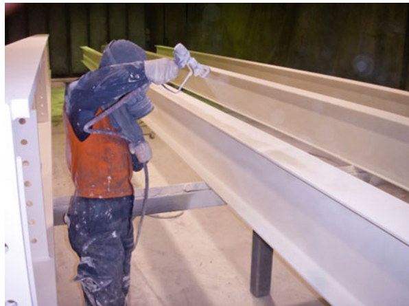
Fig. 5.11 Shop application of an intumescent coating [Image courtesy of International Paint Ltd.]
