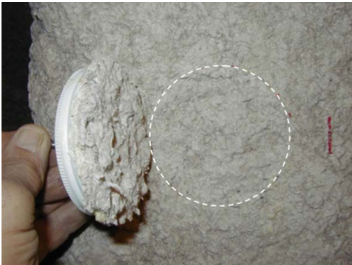
Fig. 5.13 SFRM cohesion failure (during a pull test) [25]
