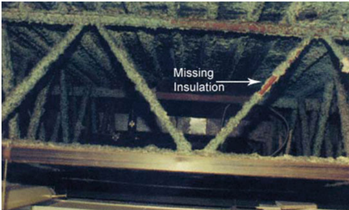
Fig. 5.12 SFRM adhesion failure (localized) [25]
