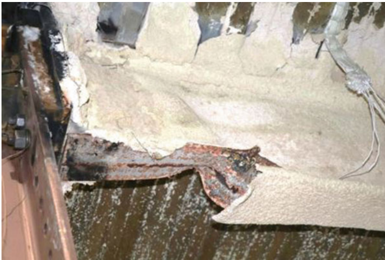
Fig. 2.6 Steel beam flange buckling
