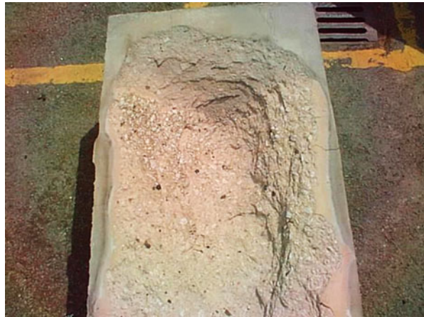
Fig. 11.27 Explosive spalling of loaded slab subject to hydrocarbon fire exposure
