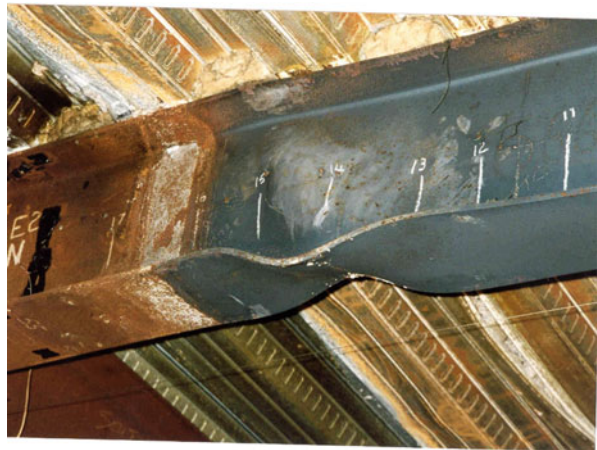
Fig. 11.9 Local buckling of beam lower flange
