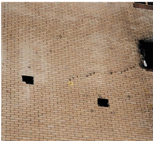
Fig. 11.43 Inclined cracks in masonry façade following a fire
