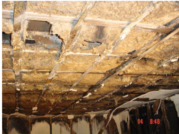
Fig. 11.15 Cold-formed steel floor following a fire
