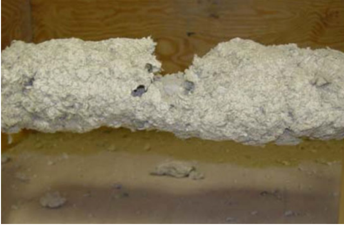
Fig. 5.14 SFRM local damage due to impact [25]
