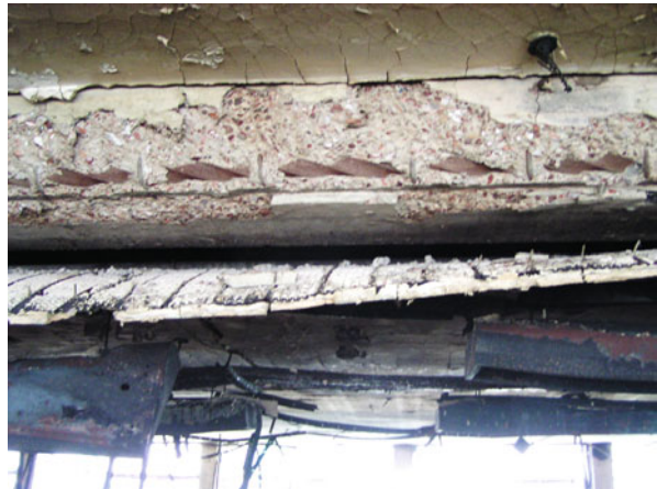
Fig. 11.31 Beam reinforcement exposed due to spalling (note: pinkish discoloration of aggregate)
