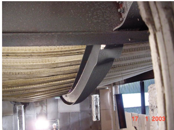
Fig. 11.7 Steel beam and composite floor slab subject to significant deformation due to fire
