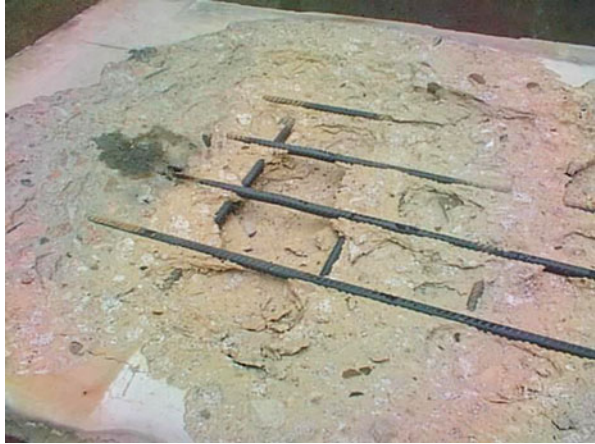
Fig. 11.28 Explosive spalling of loaded slab subject to hydrocarbon fire exposure exposing reinforcement
