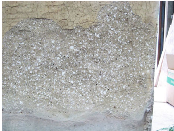
Fig. 11.25 White discoloration of limestone aggregate following exposure to hydrocarbon curve (1200 °C)
