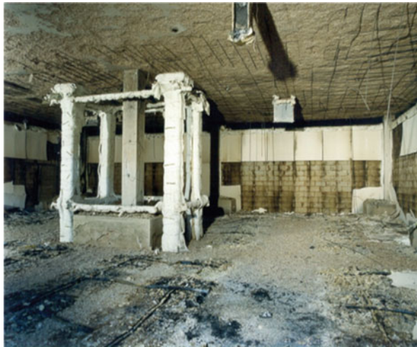
Fig. 11.29 Extensive aggregate spalling of the underside of concrete floor slab exposing tensile reinforcement
