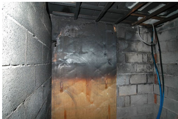
Fig. 11.4 Soot layer on oriented strand board indicative of stratification of hot smoke layer
