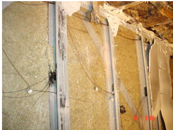
Fig. 11.16 Cold-formed steel wall panel following a fire
