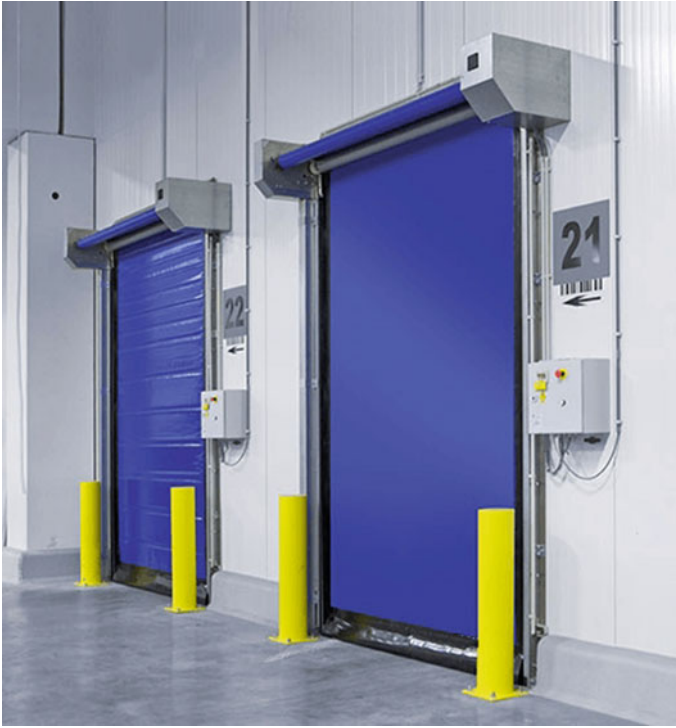
Fig. 5 Freezer high-speed doors [4]
