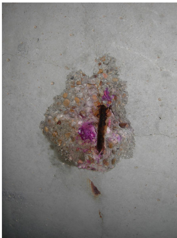
Fig. 6 Picture of the corrosion rebars in the structure A in a carbonation zone
