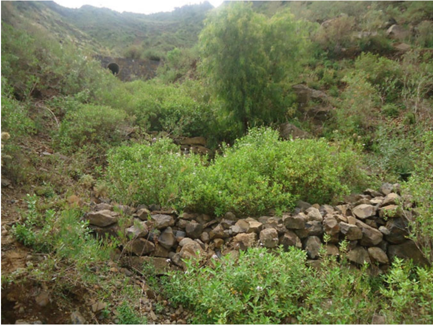
Fig. 17.6 Gully formed by road culvert; it is treated by check dam in Abiager watershed
