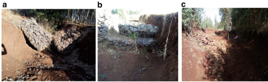
Fig. 21.6 Ineffective stone and gabion check dams on large gullies. A lack of apron (a), ineffective side key (b), and damaged stone check dam (c)
