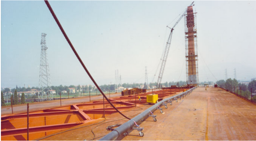
Fig. 14 The cable-stayed bridge over the Arno river. A. Montemagni, P. Sica, F. de Miranda. 1969–1978. Image during the realization (Archive “Studio de Miranda Associati”)
