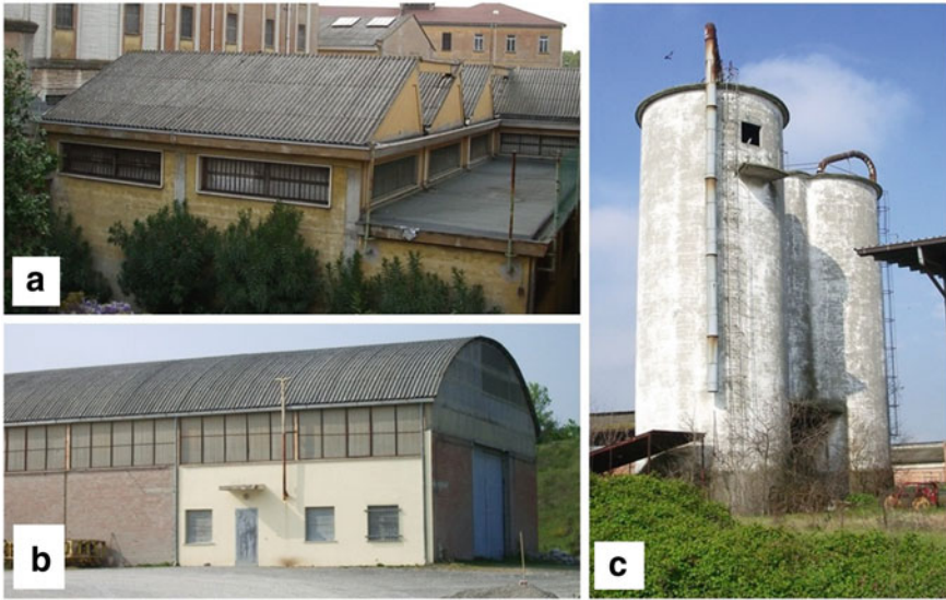
Fig. 16.2 Examples of asbestos containing building materials (ACBMs) a corrugated cement-asbestos roofing of a building in an urban industrial area; b bent corrugated cement-asbestos roofing of a building in a rural industrial area; c a grain silo in a rural area. Original pictures taken by A.F.G
