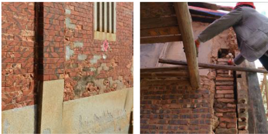
Fig. 18. Photo of a frequently-occurring issue in the wall and its repair (Shunyu Dacuo).
