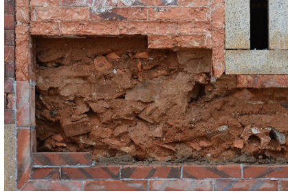
Fig. 6. Wall containing broken bricks (Shunyu Dacuo).
