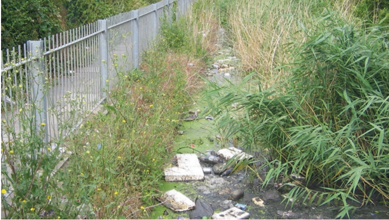
Fig. 9.2 Example of a nature-based solution with inadequate stewardship. The stewardship of this stormwater management ditch was not considered in relation to appropriate management. As such, it is seen as a negative feature of the area and is used for dumping of trash. (Photo credit: Stuart Connop)
