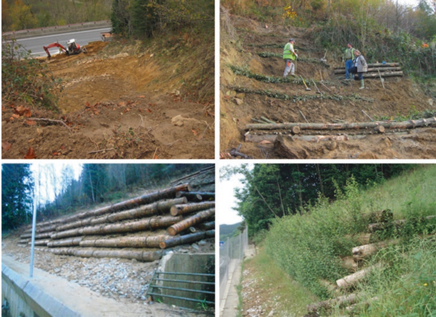
Fig. 17.5 Evolution of the work carried out on Road N1 (Guipúzcoa, Spain): comparison of images from 2011 to 2013. (Photo credit: P. Sangalli and P. Cornellini)
