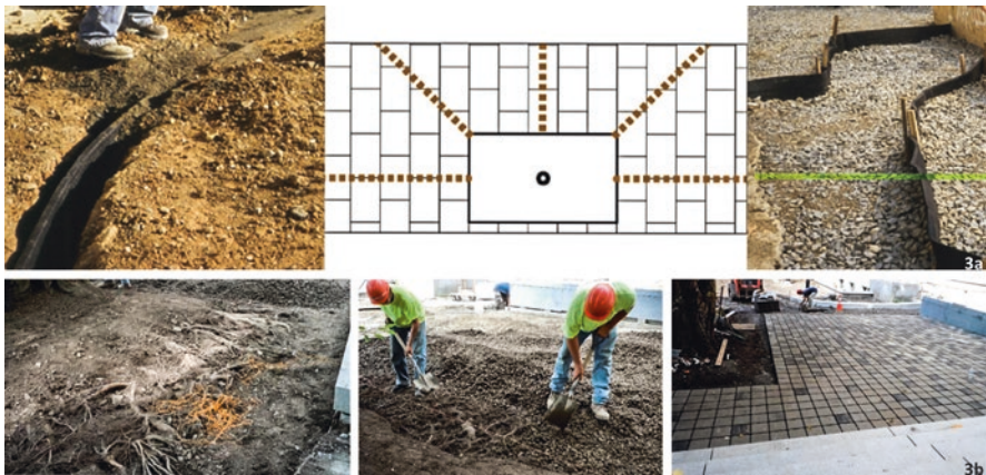
Fig. 27.3 (3a) Root path construction and schematic. (Credit: Casey Trees, Washington D.C.); (3b) Cercidiphyllum japonicum retrofit repaving with CU-Soil®. (Credit: Urban Horticulture Institute Cornell University)
