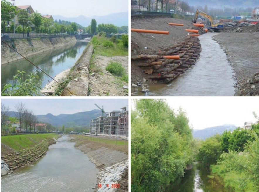
Fig. 17.3 Evolution of the work carried out on Artía Channel (Spain): comparison of images from 2002 to 2019 (i.e. after 17 years of service life). (Photo credit: P. Sangalli)
