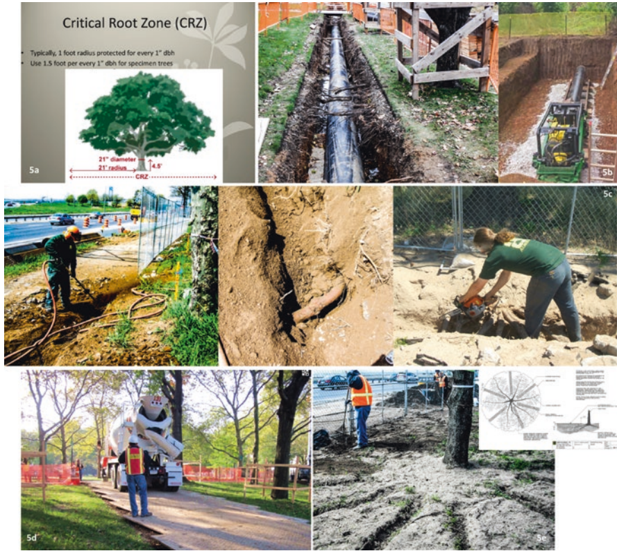
Fig. 27.5 Building WITH Trees: (5a) Planning – CRZ (Credit: Urban Hort Inst.); (5b) Design – Trenchless technology (Credit: C. Glaeser); (5c) Pre-Construction – Pneumatic excavation + root pruning (Credit: C. Glaeser); (5d) Construction – Ground protection mats (Credit: C. Glaeser); (5e) Post Construction - Radial trenching + detail. (Credit: C. Glaeser, N. Zürcher)
