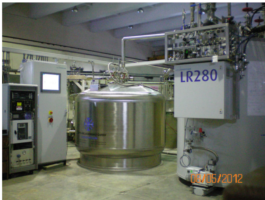
Fig. 1.8 Modern-day turbine-based helium liquefier with a refrigeration capacity of 900 W (~300 L/h) manufactured by Linde Kryotechnik AG installed at IUAC in 2012. Photo courtesy IUAC Delhi
