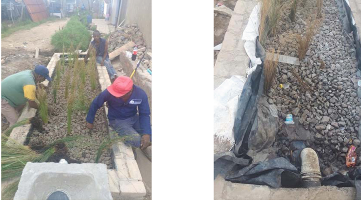
Fig. 2. Constructed wetland just before final installation (left) and after four months (right).
