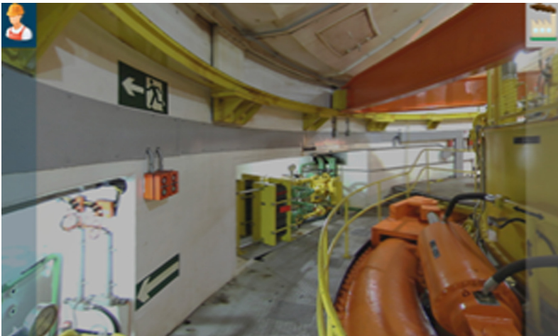
Fig. 3. Power plant navigation: access point to heat exchangers.
