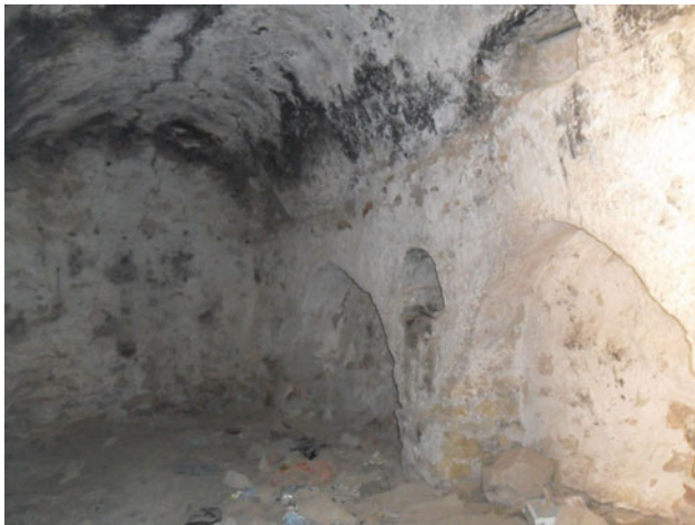
Fig. 7.4 Cracked vault (Author's photo)
