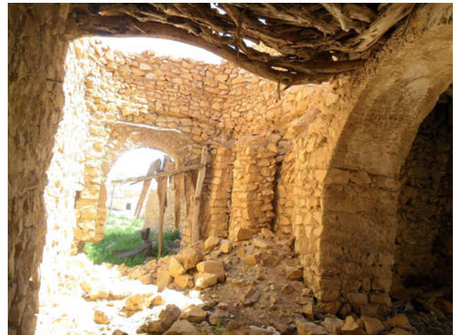
Fig. 7.5 Degraded flat roof (Author's photo)
