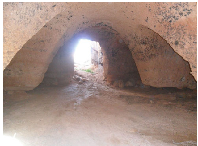
Fig. 7.8 Disappearance of a part of the walls (Author's photo)
