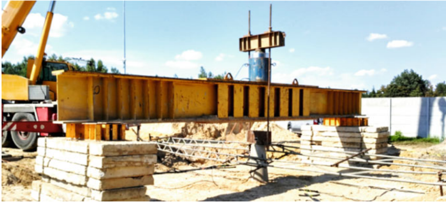
Fig. 11 The view of the stand for pulling the footing out from the ground
