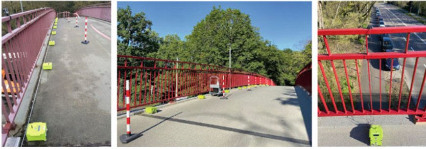
Fig. 5 left : Sensor positioning before the renovation; center : Sensor positioning after the renovation; right : Menhir with GPS antenna
