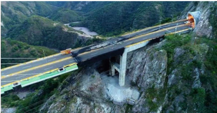
Fig. 3 View of the El Carrizo Bridge the day after the accident
