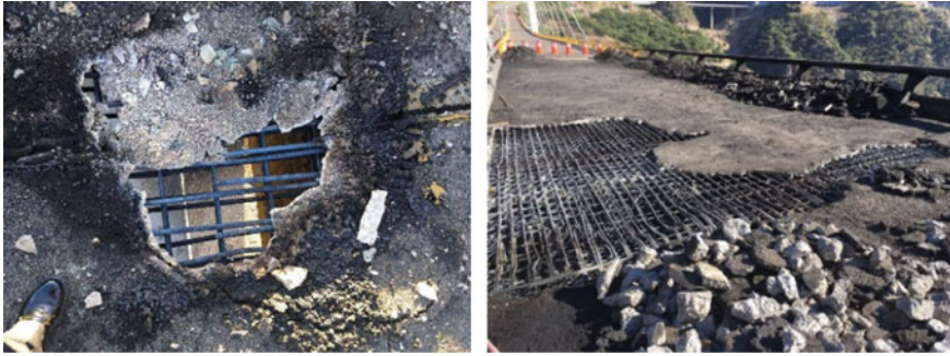
Fig. 4 Some details of the damage caused to the bridge deck
