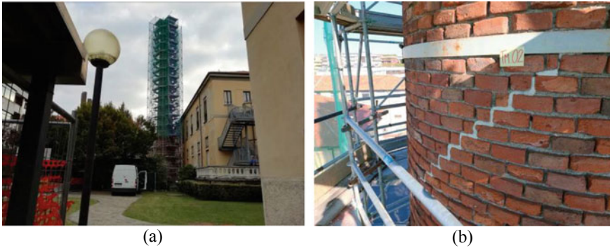
Fig. 1 a A general view of the structure with the temporary safety scaffolding and b a detail of the outer masonry layer
