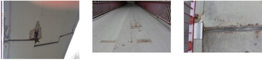
Fig. 4 left : Corrosion damage on the eastern support console; center : Corrosion plums in the support area; right : Corrosion plums on the expansion joint
