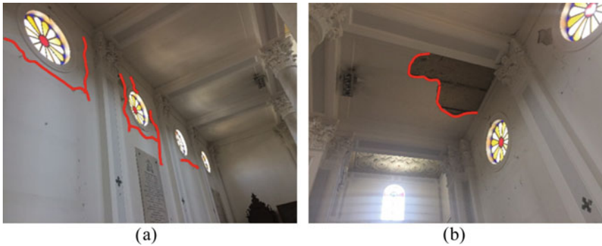
Fig. 3 a Distribution of spread shallow cracks along the longitudinal walls of the main part of the church, b particular of the ceiling detachment
