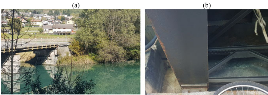
Fig. 3 a View of the right embankment to access the bridge; b detail of rust signals
