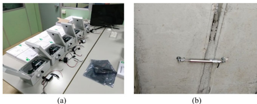
Fig. 8 a Data acquisition units in the test room; b installation of LVDT across a deck transversal gap
