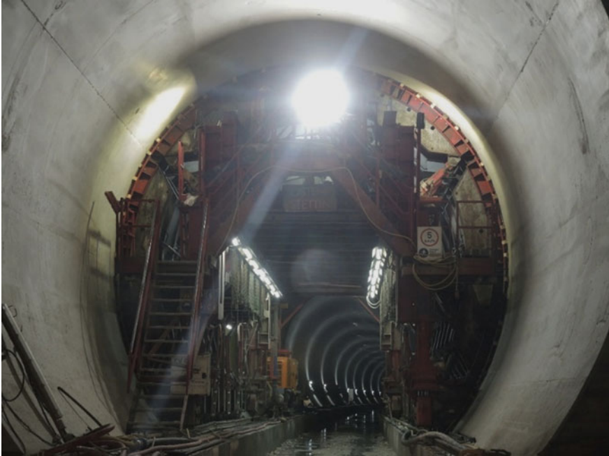
Fig. 6 Formwork platform made of steel for the construction of the concrete inner lining
