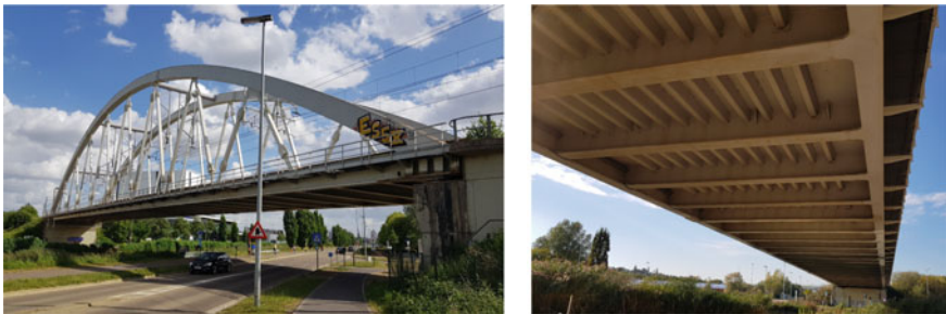
Fig. 1 The KW51 bridge, (left) as seen from the north side, after retrofitting, and (right) view on the bridge deck from below
