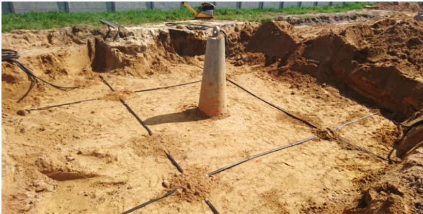
Fig. 10 The view of the 3DSensor’s arrangement within the second layer: installation stage
