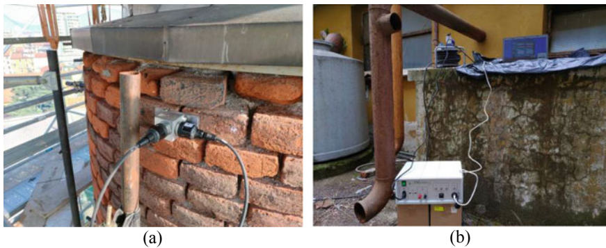
Fig. 5 Dynamic tests: a piezoelectric accelerometers on the top of chimney and b data acquisition system
