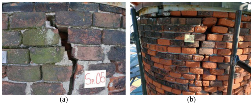
Fig. 3 Damage identification: a–b typical passing-through crack and b washout of mortar joints on the top of chimney
