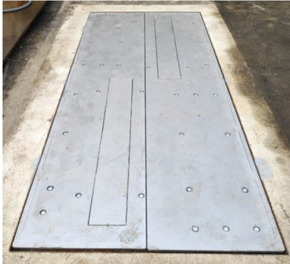
Fig. 1 The P-WIM system as it appears once installed
