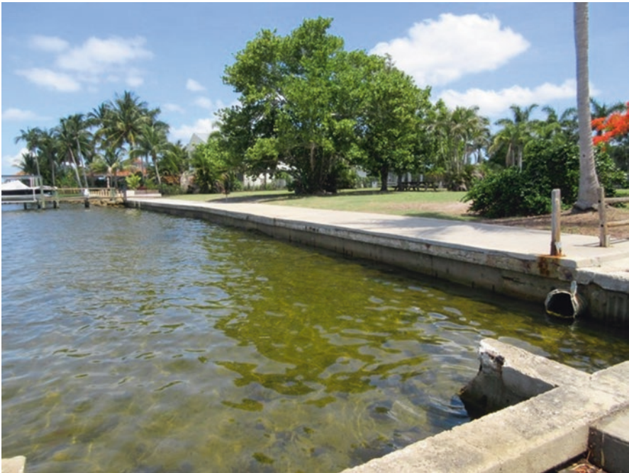
Fig. 12.6 The low sea wall along the southern shoreline of Cape Coral would provide only minimal protection from tidal surge inundation. (Source: Photo taken by the author)
